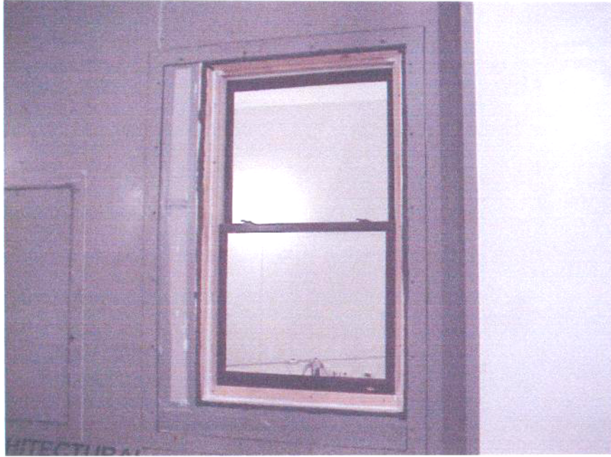
Receive Room View of the Prime Window Installed in the Filler Wall
