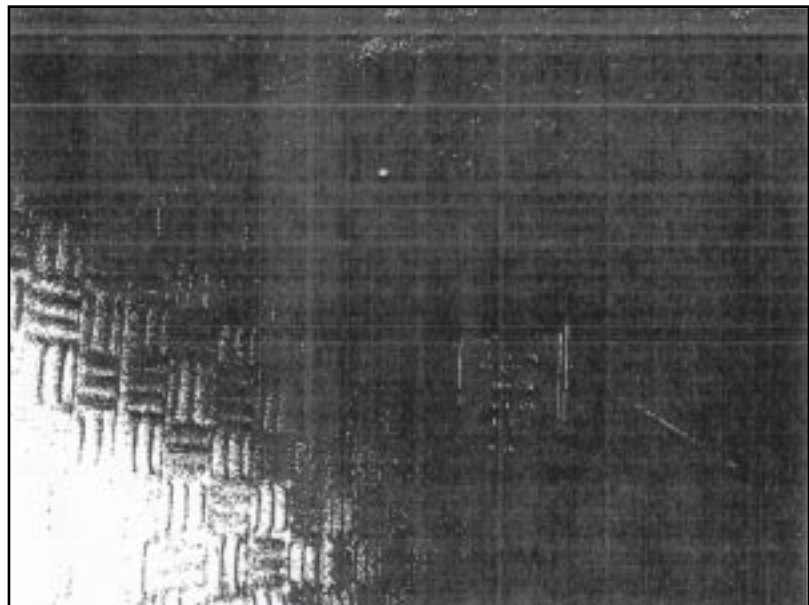
PHOTOS 4. 12 ft. Wall Charring
